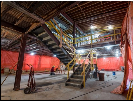
December, 2019 – This photo shows the interior stairwell in the open foyer (between main & 2 nd floor).
